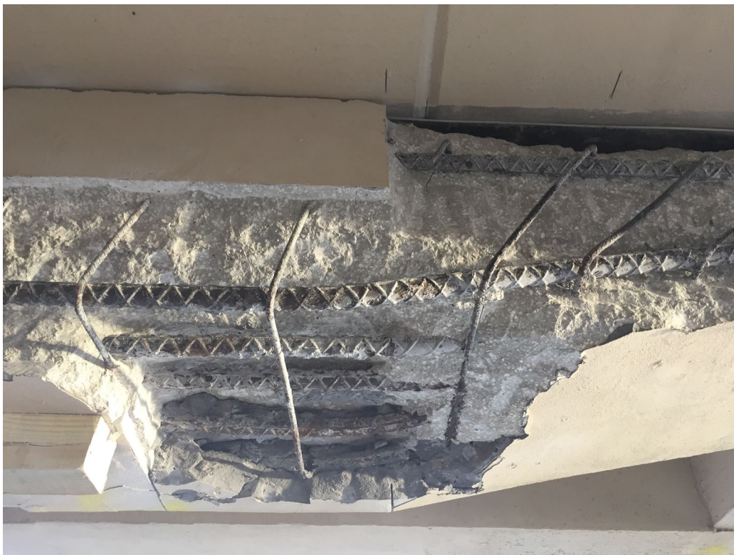
Picture 4: Repair still cracked, requires further chipping
